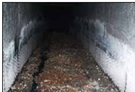
Discharge flume with damaged tile/rubber liners.
