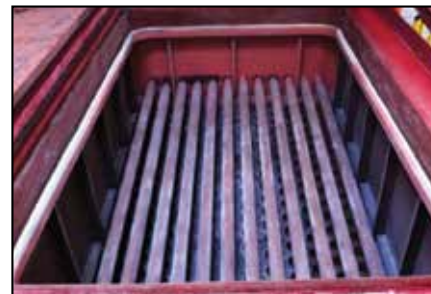
Bag house protected with ARC S7 in service over 2 years with no failures.
