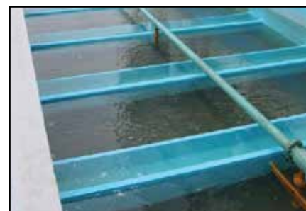
Sand filter in service.
