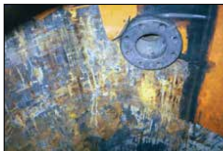
Removal of the rubber lining in progress. Blistering of the lining is visible.
