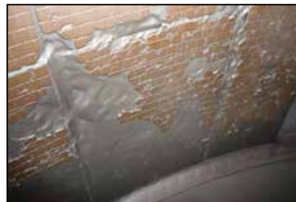
Damaged pulverizer walls.
