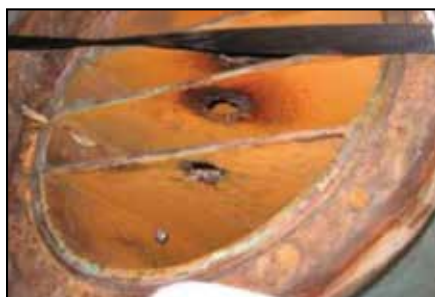
Corroded divider plates.
