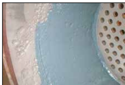
After application of ARC 858, ARC SD4i is applied for protection and enhanced flow efficiency.
