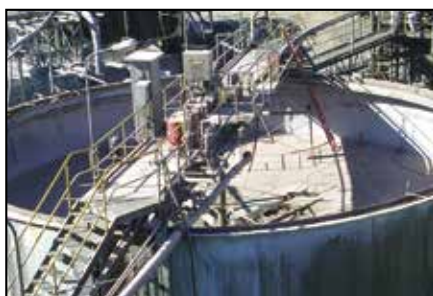
Slurry thickener at a major South American mine.
