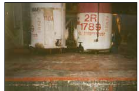
ARC 988-coated floor areas.
