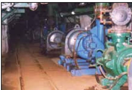
Bank of dewatering pumps.
