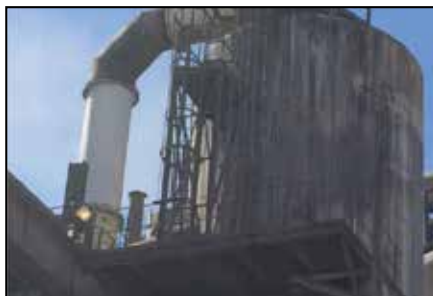
Flash cooler with exhauster.
