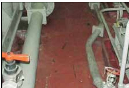
Previous coating one year after installed.
