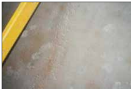
Corrosion and pitting on the spillway gate.
