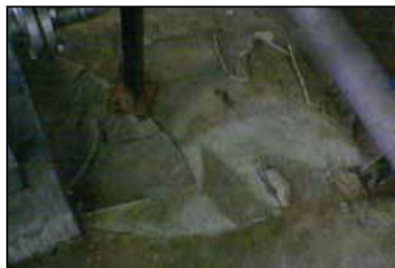
Delaminated fiberglass mat polyester.
