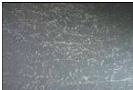
Corroded tank internal surface.
