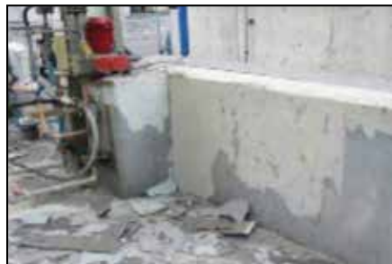
Failed coating after spills.
